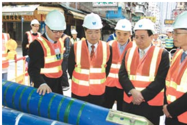
Mr Nicholas NG (second left), Chairman of the Public Service Commission, Mr Nicky LO (first right) and Mr Vincent LO (third right), Members of the Commission, accompanied by Mr MA Lee-tak (second right), Director of Water Supplies, visited a work site in Shamshuipo of the Water Supplies Department.
